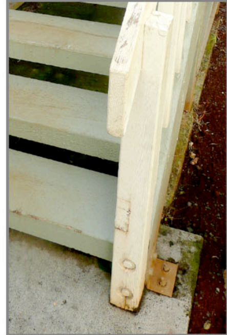
Above is "Before" at a different Waipio condo, but same original builder. These posts and stringers had deteriorated to the point they all needed replacing.
