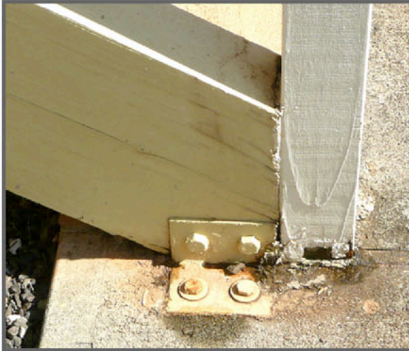
Above post & stringer clearly needs replacement. This may be one of the few in the project that needs such major work. (next time, put brackets on the inside.)
