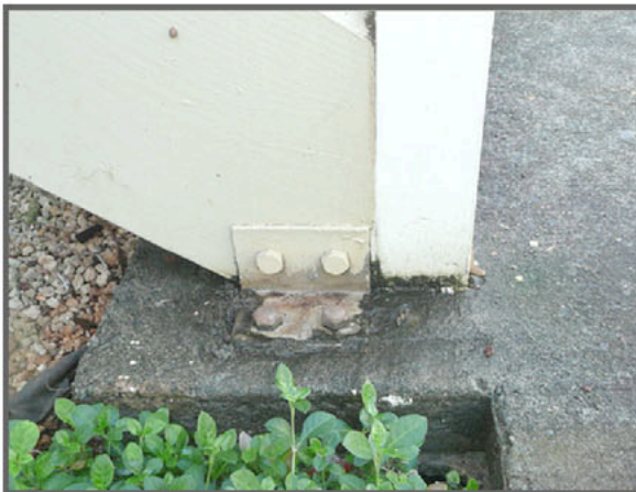
Above is typical of generally well-maintained stringers and posts in the same project as top. When tapped or poked, they sound solid, so probably don't need replacing. Water hasn't wicked up from the slab and done more than cosmetic deterioration, so treat at the same time the stair treads are replaced. Some angles may have to be replaced, but not these.
